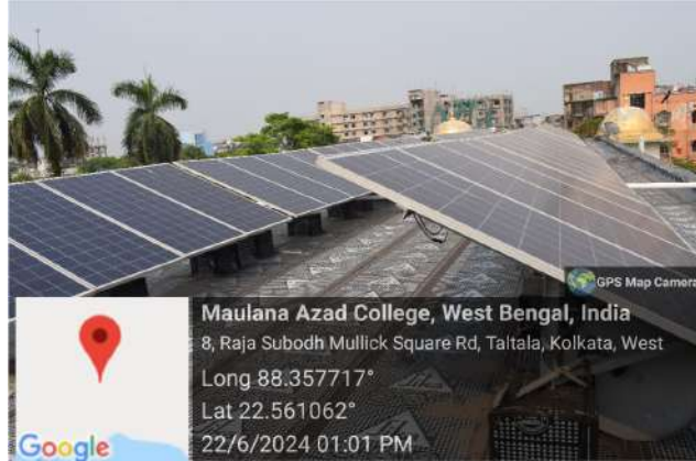
Rooftop Solar Panel
